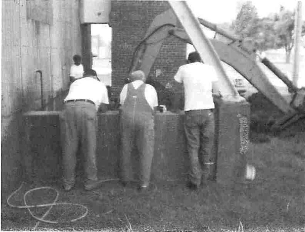
The DAM crew (left to right: Amos Page, Martin Moyer, Dale Allen) show us their best sides as they supervise the excavation of a sewer line outside Hangar 604.
